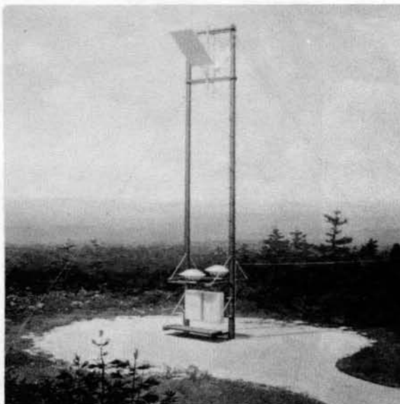
REPEATER STATION UTILIZING H - FRAME TOWER
